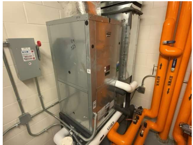
16 - GROUND SOURCE HEAT PUMP
