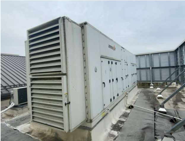
19 - EXTERIOR AIR HANDLER
