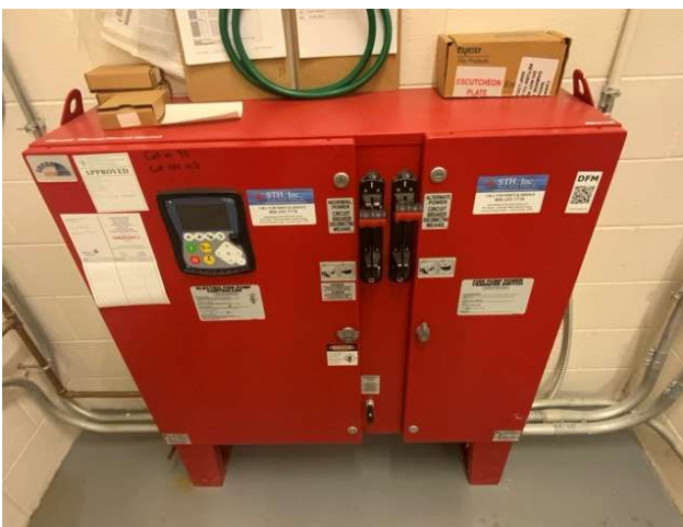
23 - FIRE PUMP CONTROLLER
